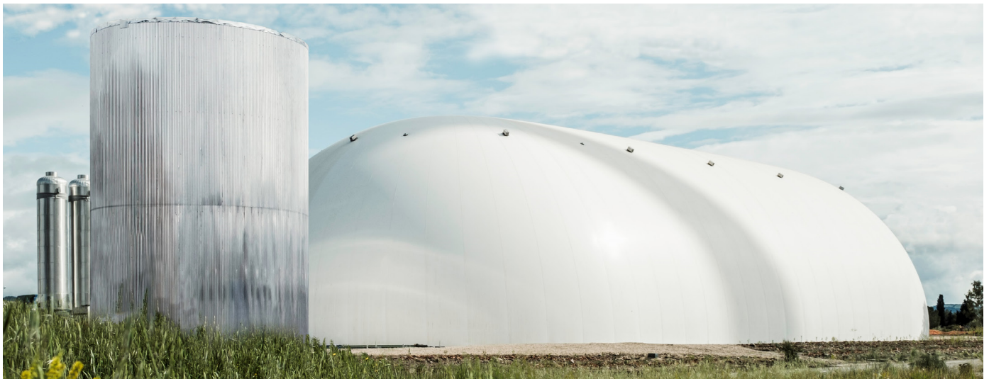
Energy Dome's CO 2 battery located in Sardinia, Italy.
