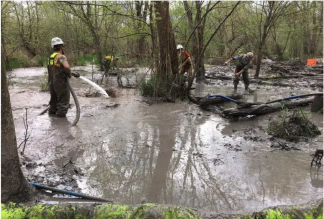
Figure 3. Workers clean up following an HDD inadvertent release of approximately two million gallons of drilling fluid into a wetland while drilling under the Tuscarawas River as part of the Rover pipeline project in Ohio (Photos source: Ohio EPA, 2017).
