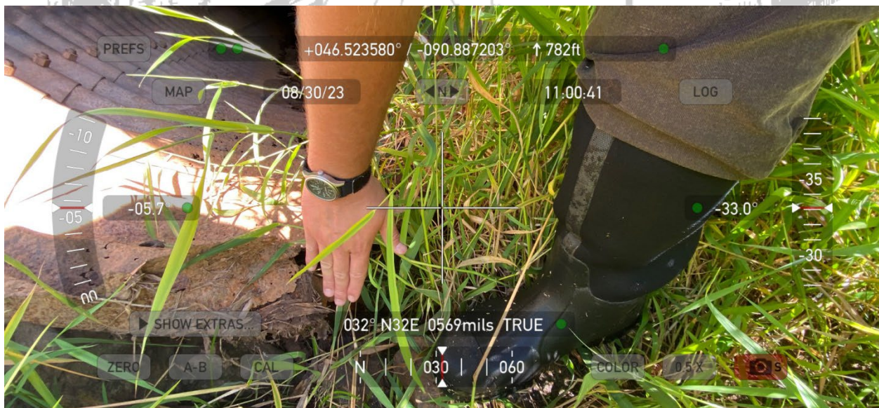
Figure 12. MNRD staff at the crossing for Beartrap Creek at Hegstrom Road where the pictured culvert was approximately 9 inches above the surface of the creek.
