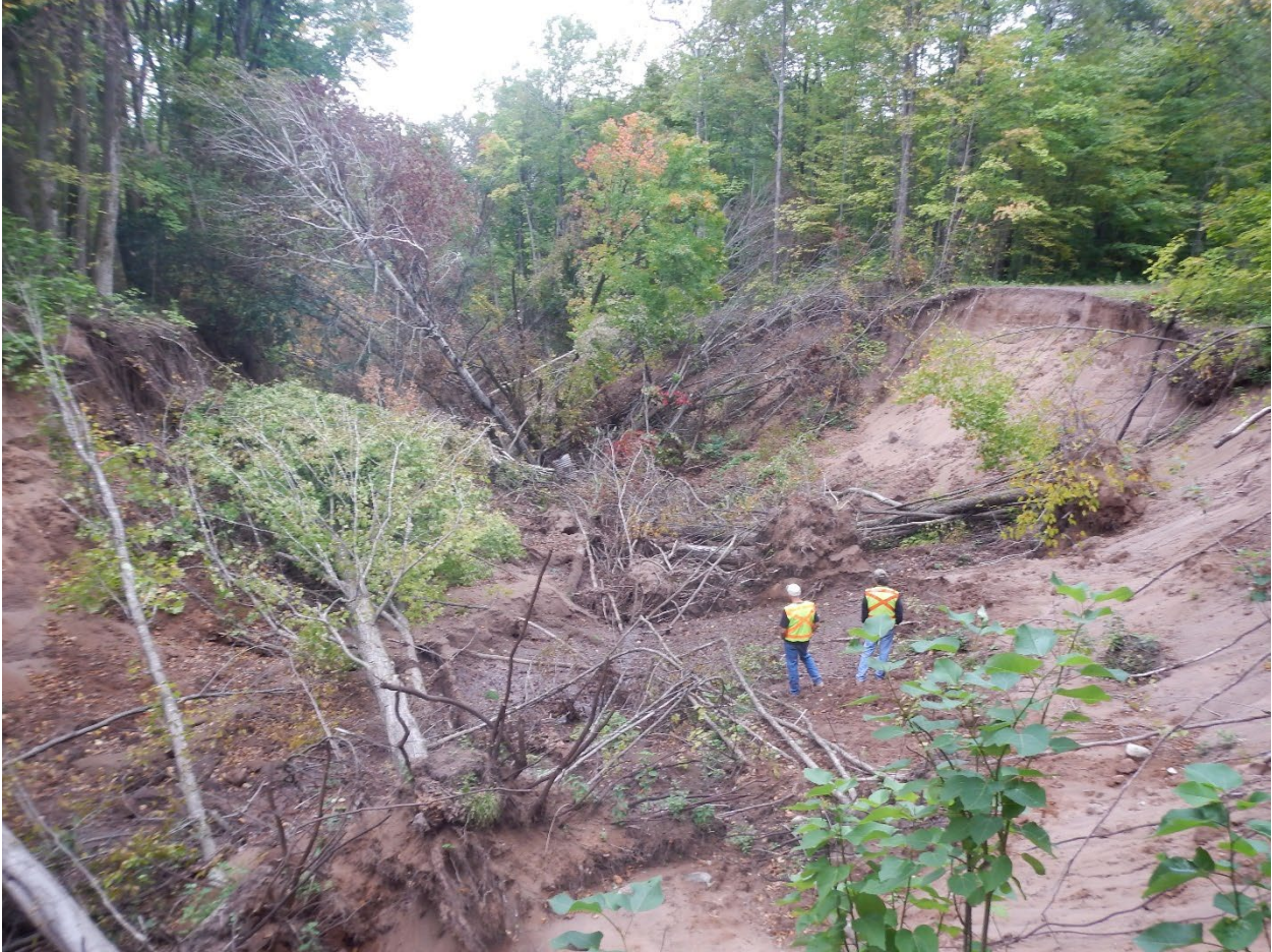
Figure 4. Winks Creek, a cold water trout stream within the Bad River Reservation, was impacted during the July 2016 flood by elevated groundwater and surface water flows. Photo showing washout of Winks Creek taken on September 20, 2016 by MNRD staff.
