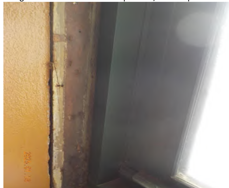
Example of original window casement in Kitchen Shown #24 – pickable/cracked paint
