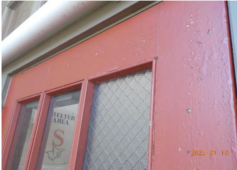
East Lobby off 3-G1 stairwell – left interior door blistered/ chipping paint.
