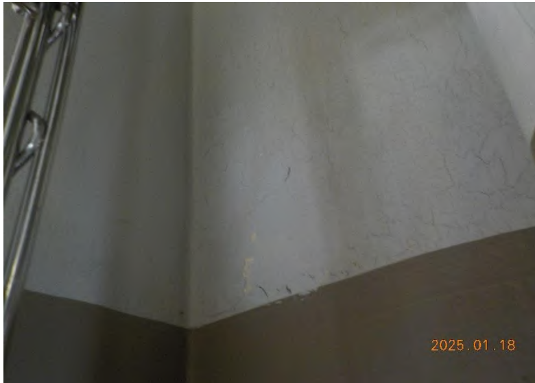
Kitchen Receiving – wall C (south) – spiderweb cracks/minor chipping
