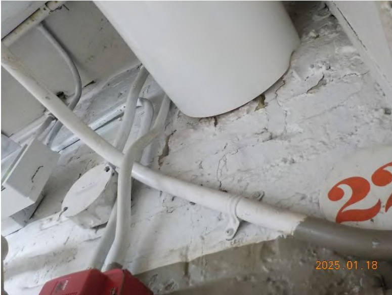
Corridor G-1A (outside kitchen) – upper wall left of drinking fountain. Chipping/flaking paint.
