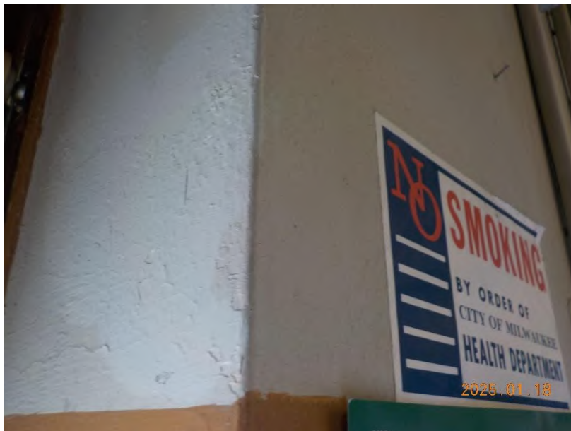
Kitchen – wall C (south) – spiderweb cracking/chipped paint
