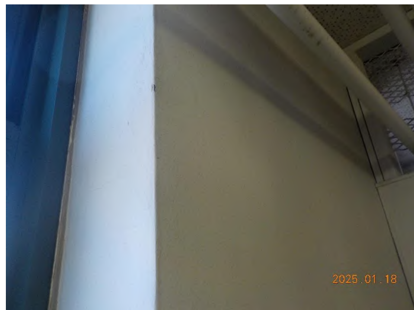
Kitchen Receiving – wall D – spiderweb cracking/minimal chips
