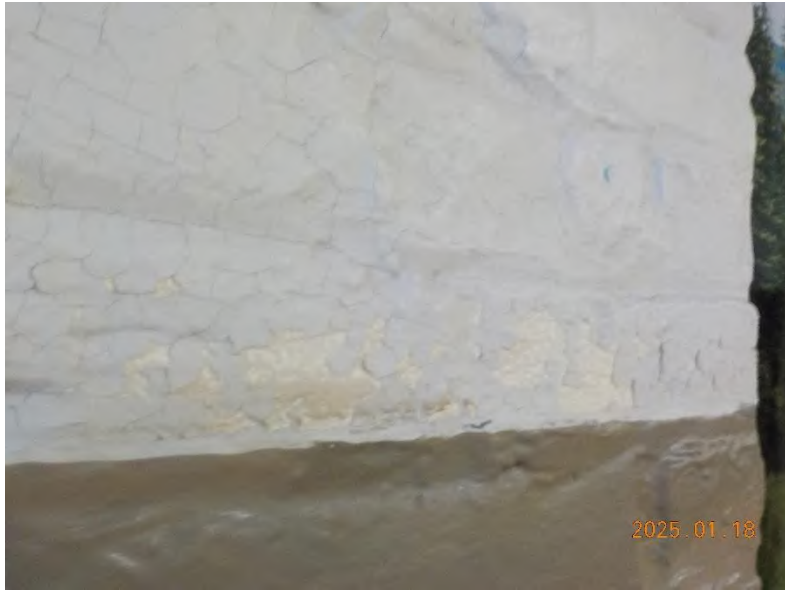
Teacher's Lounge – wall A (north) – spiderweb cracking/flaking
