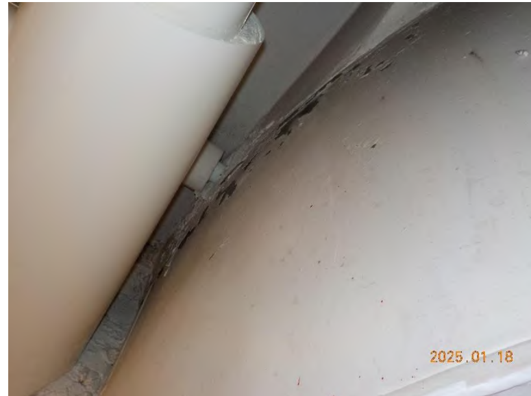
Corridor G-1A HVAC ductwork above drinking fountains. Chipping/flaking paint.
