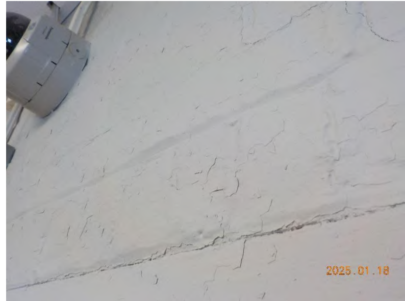
Teacher's lounge – wall B (east) – spiderweb cracking
