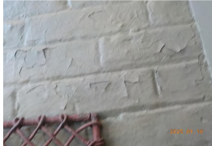
Walls A (north) & C (south) of East Lobby have blistered/peeling paint.
