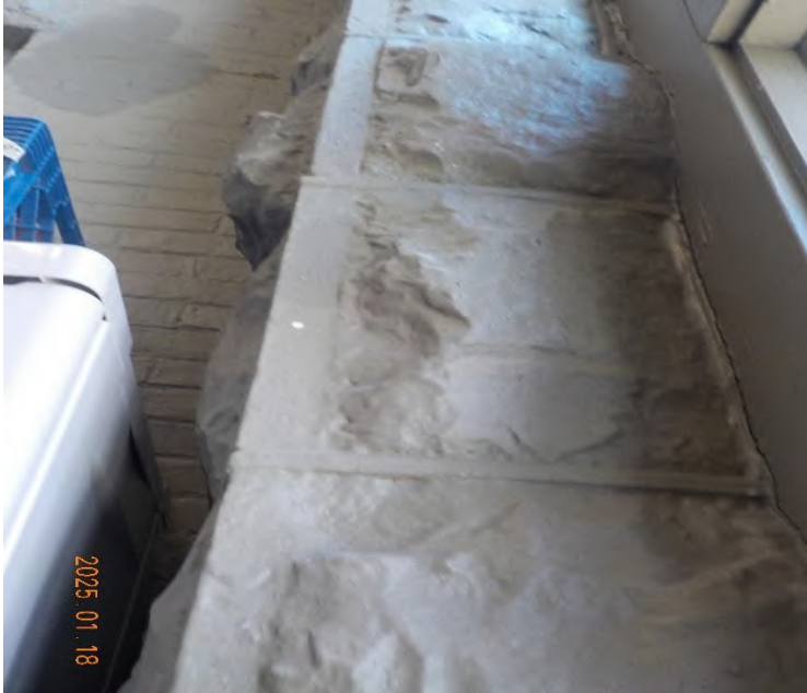
Stone masonry column north (left) of exterior doors inside East Lobby – blistered paint that chips easily if touched
