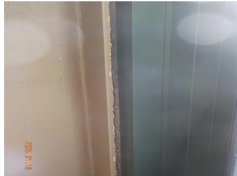
Example of original window casement(trim) in Kitchen Receiving along walls C & D - Shown #25 – pickable/cracked paint
