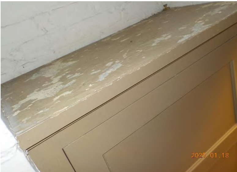
Teacher's lounge (G-08) storage cabinet (by entrance) – top surface. Paint chips can easily be dragged off if items stored here.
