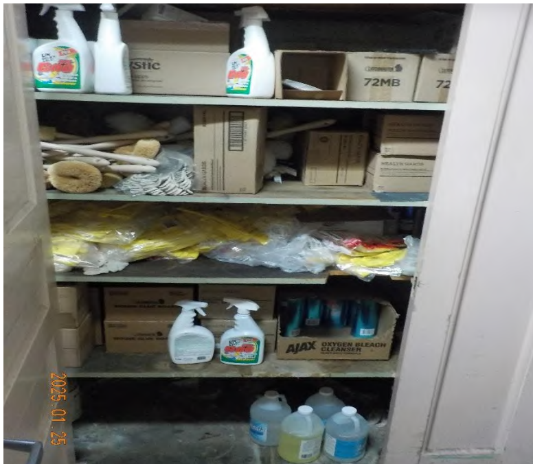
Wall C cabinet – shelves (all) – chipped paint
