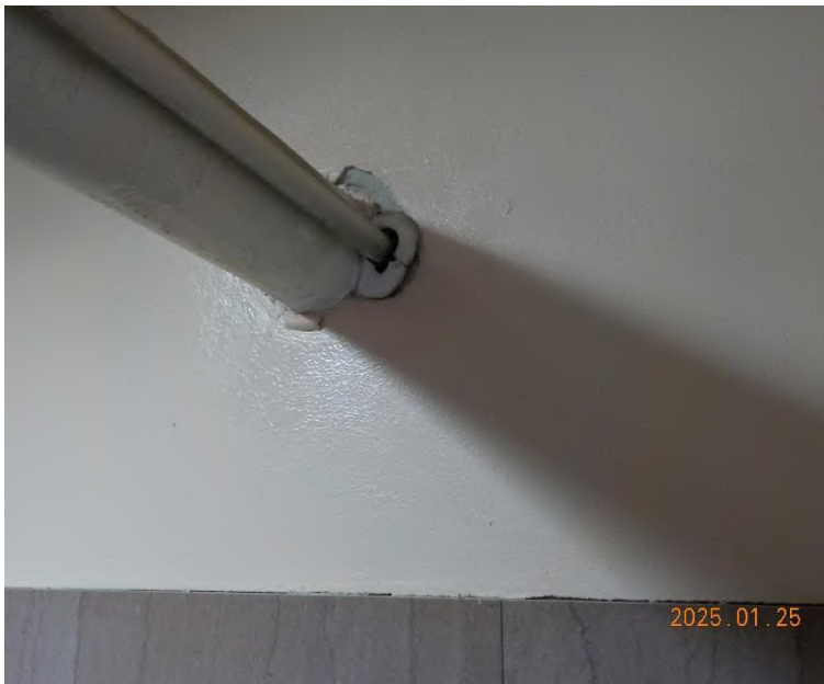
009 – West wall B of toilet area – (cracks/chipping around pipe)
