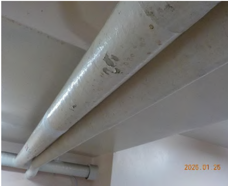
GB 009 – system pipe along ceiling in sink area (peeling paint)
