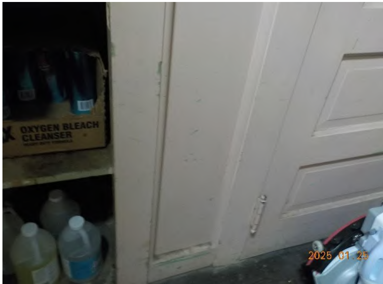
[Janitor's room] 007B -wall C cabinet frame deterioration (chipped)
