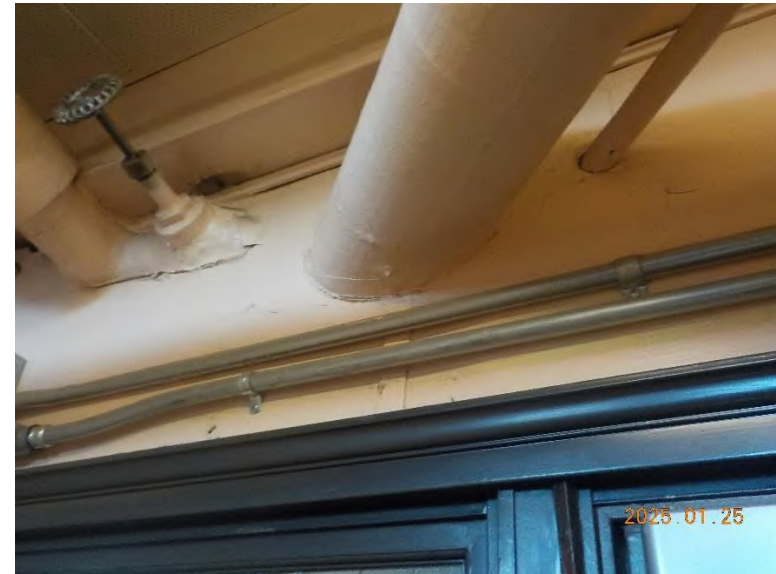
Stair 2-G1 – North wall deterioration over doors (cracking)
