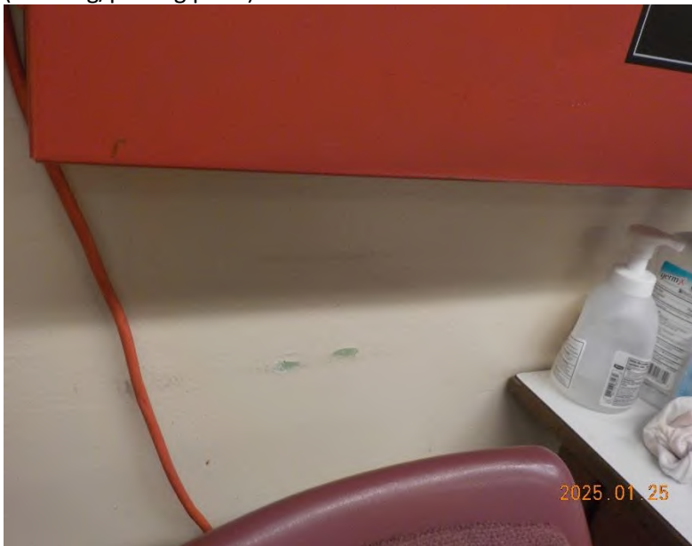
Room 003 East wall D (cracking & friction damage)
