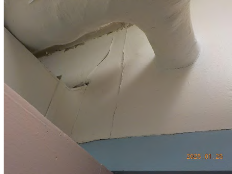
Rm 008A – North Wall C (cracking)
