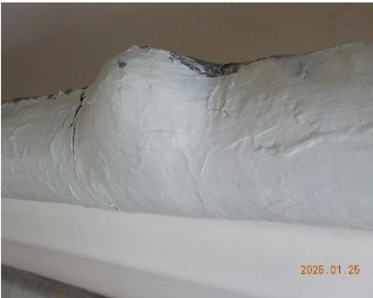
Rm 002 system pipe along ceiling by (east) wall D (cracking)
