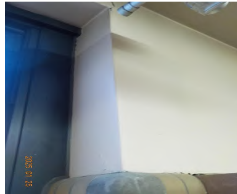
009 – North wall C by toilets (cracked/chipped paint)
