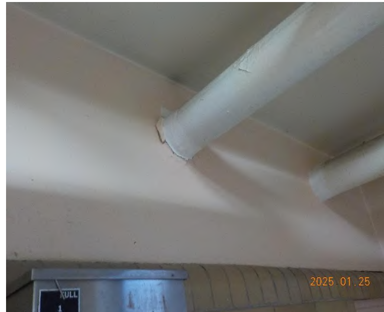
009 – North wall C over sinks – (cracked paint around pipes)
