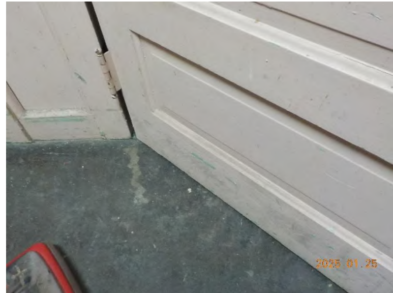
Wall C cabinet doors (all) – chipped/pickable paint
