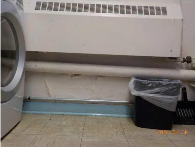
Room 008A – South Wall A deterioration (cracking/peeling)
