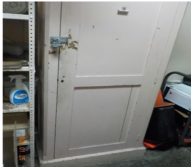
Wall A single cabinet – frame & door deterioration (chipped paint)
