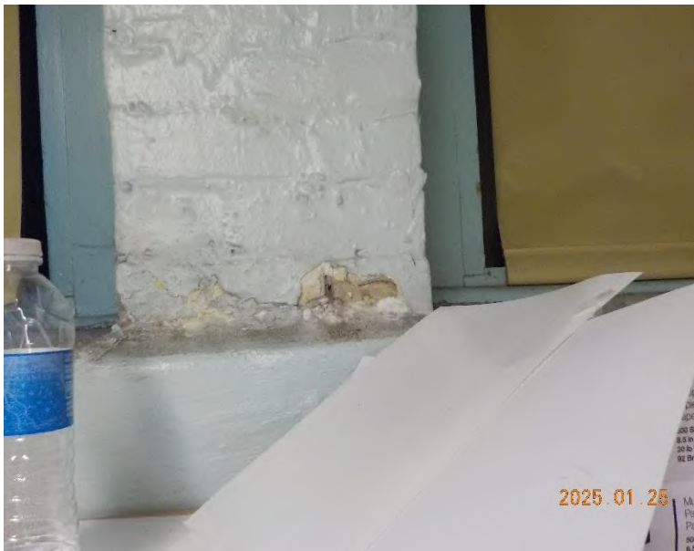
Room 006A – North wall C deterioration (cracked/chipped paint)
